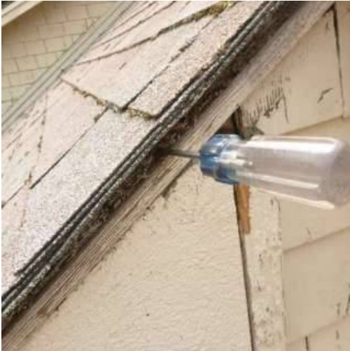
Photo 16-1 Fungal rot, roof sheathing, West side.
