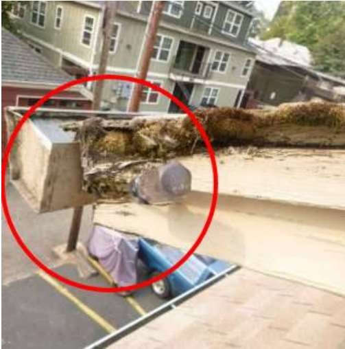
Photo 16-2 Fungal rot, barge trim board.
