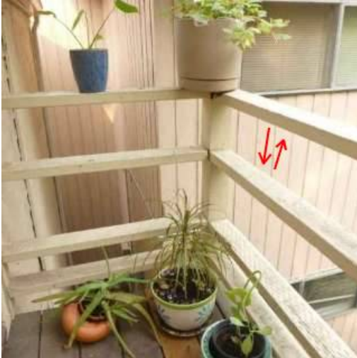
Photo 2-1 Guardrail and handrail at second floor apartment does not meet current codes.
