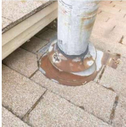
Photo 18-2 Recommend replacing all significantly corroded flues and flashings at next roofing.
