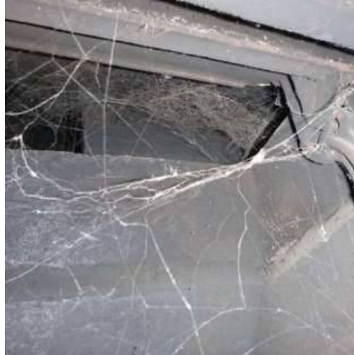
Photo 27-2 Damper was functional.
